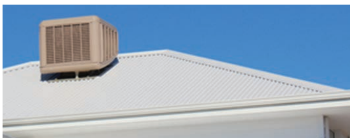
Fig. 18: Typical example of air conditioning unit screened from public view.
