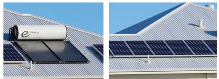
Fig. 20: Typical example of solar collectors matching roof profile.
