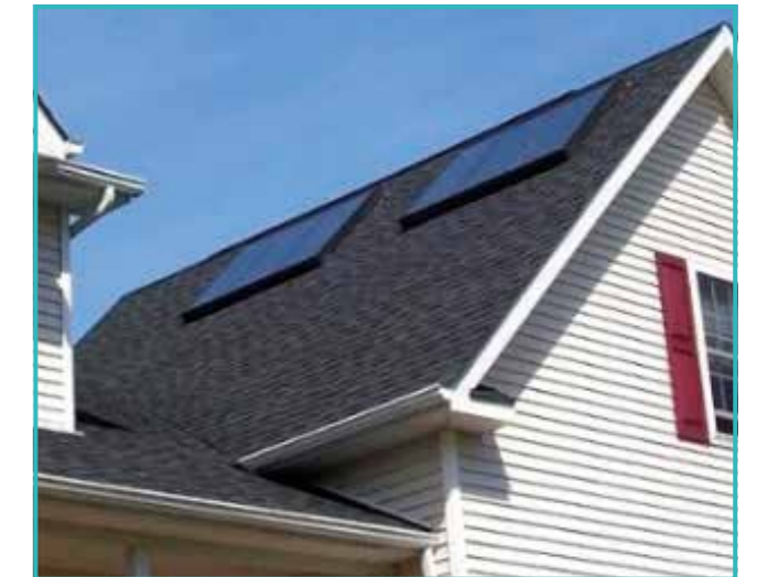
Roof-mounted solar heating
