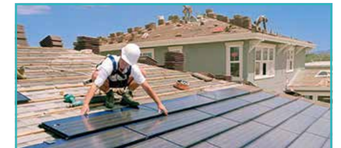
Roof integrated photovoltaics replacing roof material
