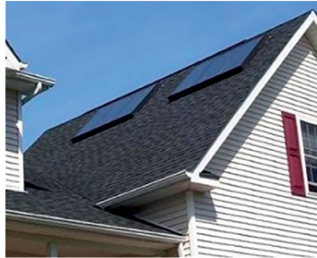
Roof-mounted solar heating
