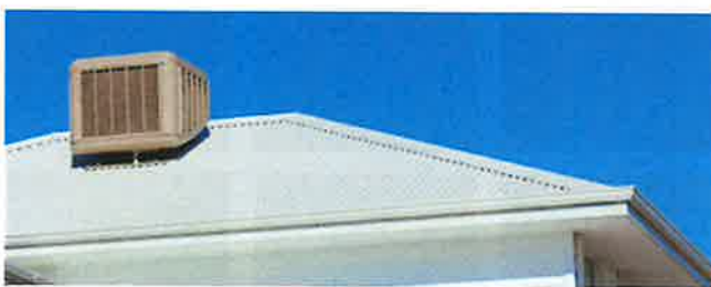
Fig.27:Typical example of air conditioning units screened from public view.
