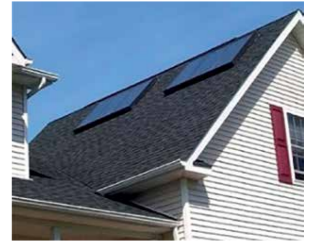
Roof-mounted solar heating
