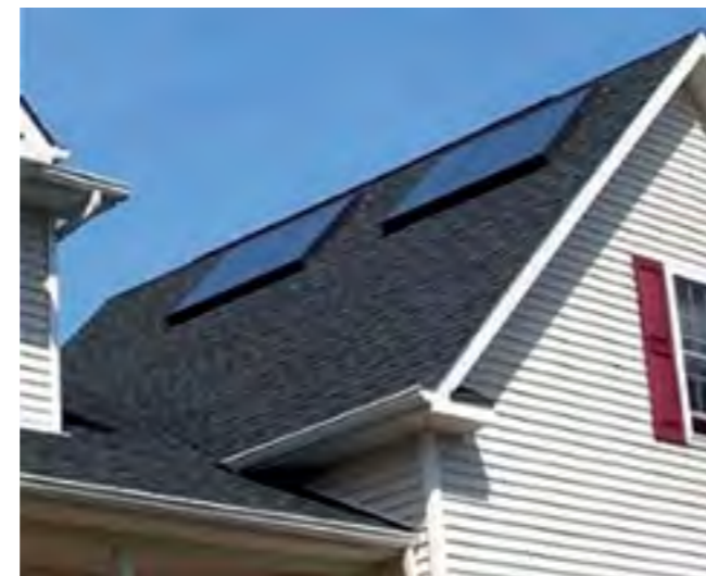
Roof-mounted solar heating
